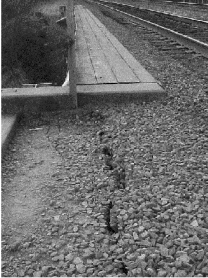
Figure 4. Settlement at bridge end at MP 31.6.
