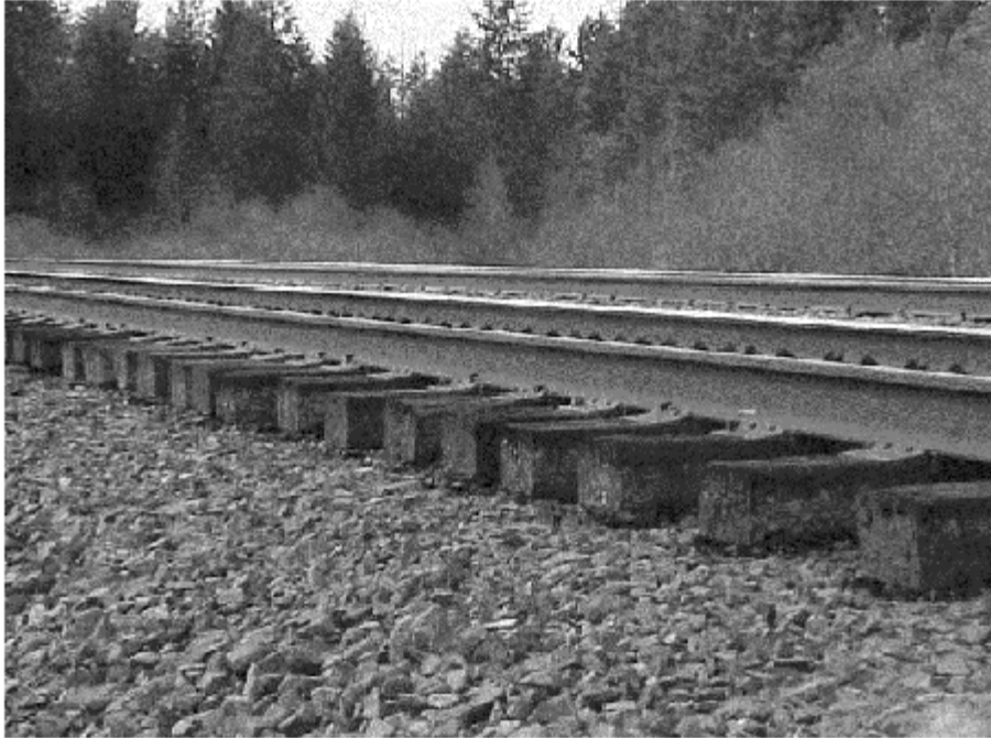
Figure 2. Settlement under track at MP 30.9.
