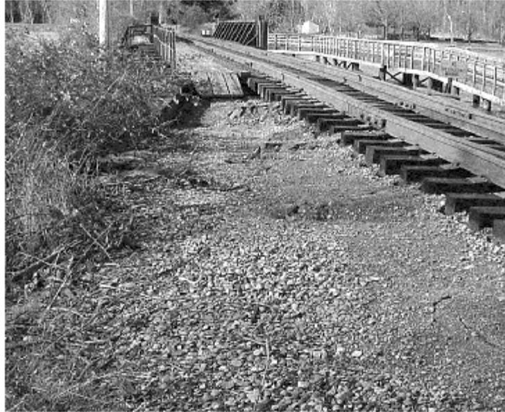
Figure 6. Settlement at bridge end at Capitol Lake.
