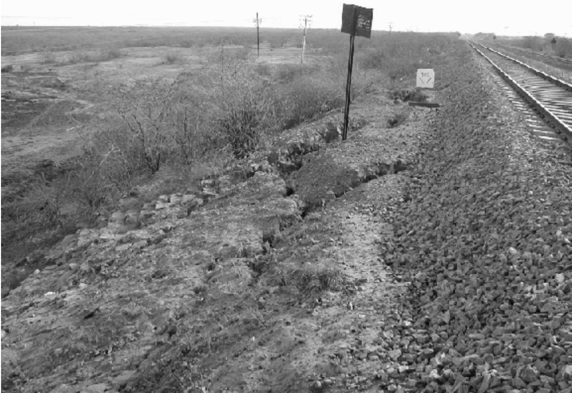
Figure 3. Cracks in embankment due to lateral spreading.
