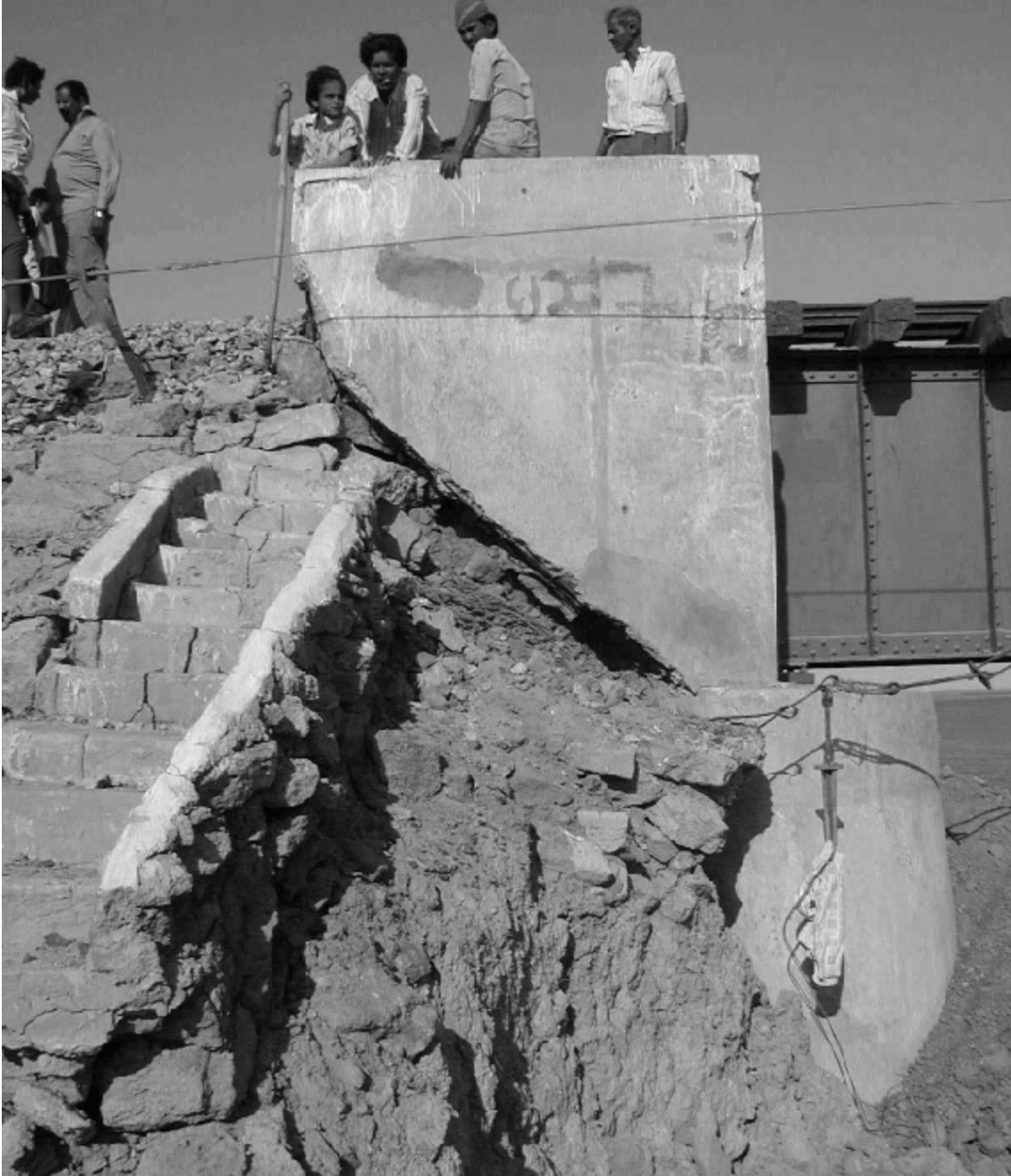
Figure 4. Settlement at Bridge No. 279
