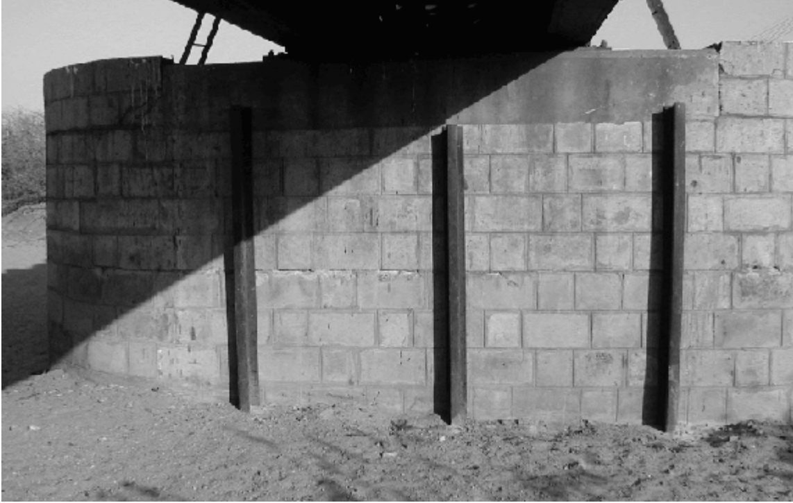
Figure 12. Rails set in concrete to resist movement of portion of pier above horizontal crack until epoxy is injected into joint
