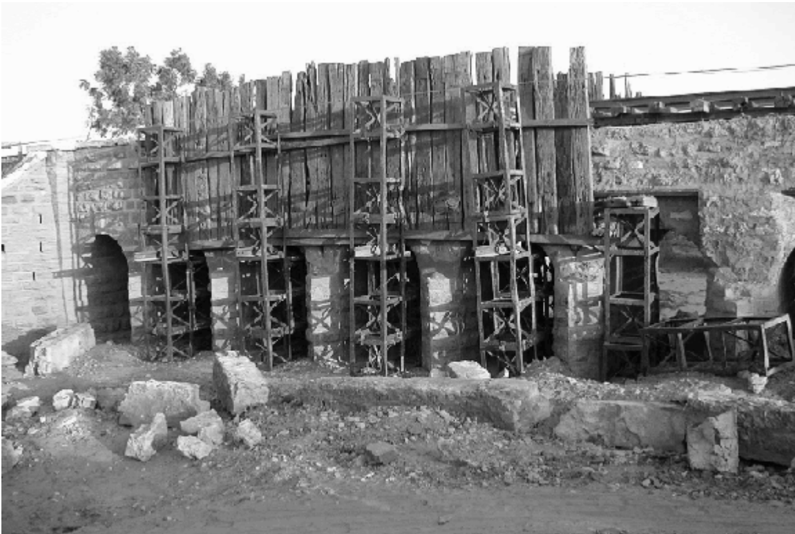
Figure 11. Shoring to retain spandrel fill and rail cluster falsework at Bridge No. 245
