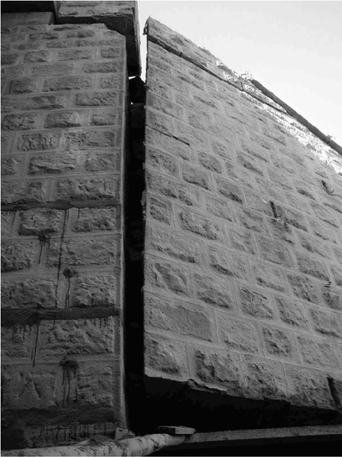
Figure 7. Wing wall separation at Bridge No. 271
