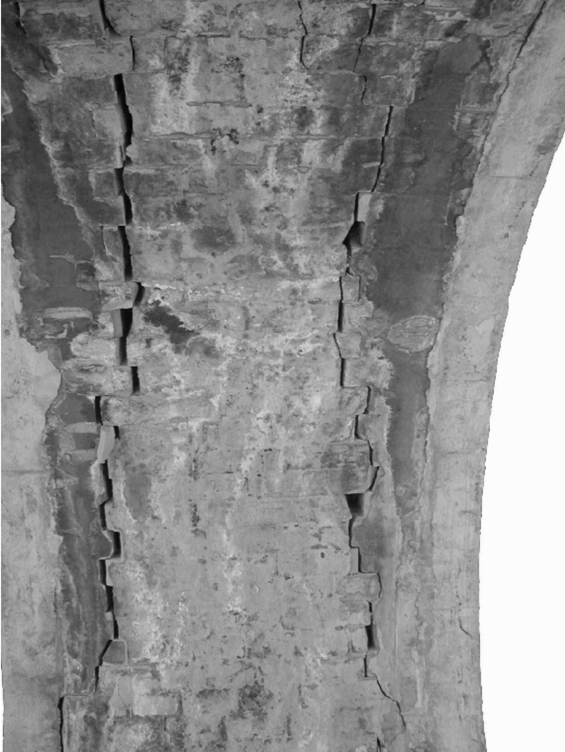
Figure 9. Separation along longitudinal joints in arch at Bridge No. 48
