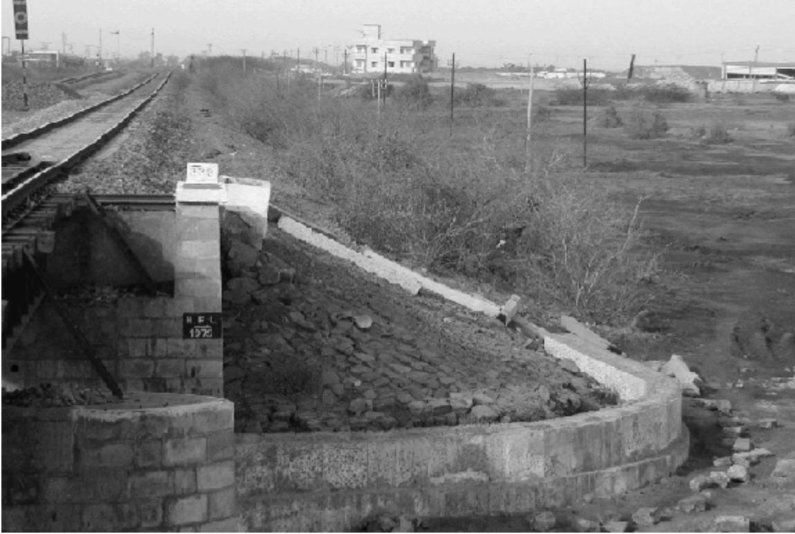
Figure 5. Settlement at Bridge No. 161
