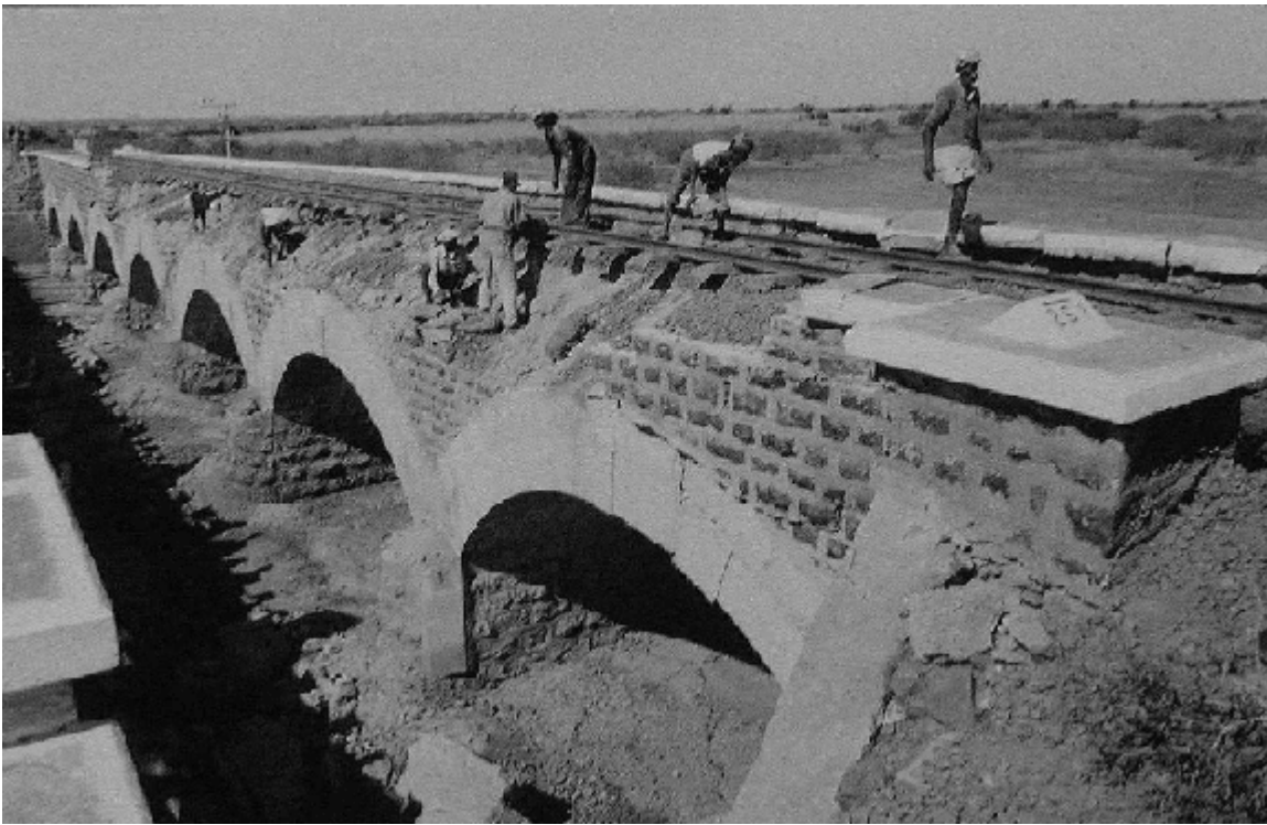
Figure 6. Failed parapet and displaced stone in arch ring at Bridge No. 261 (Western Railway photo)
